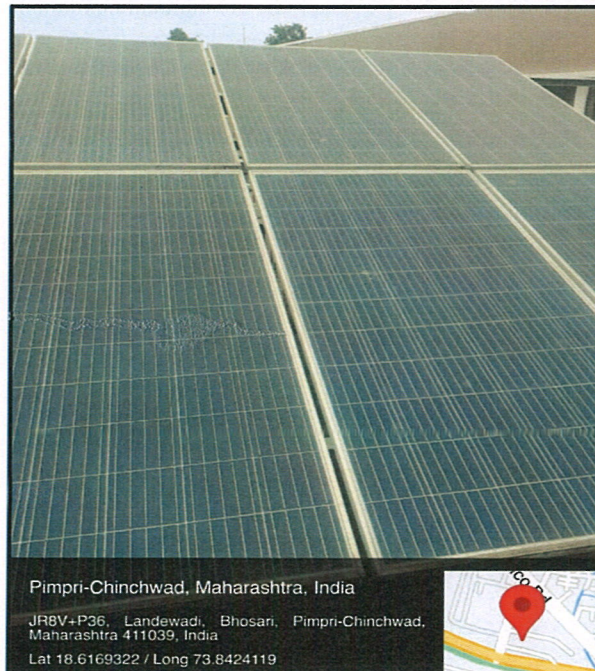
Photograph of Roof Top Solar PV Plant:
